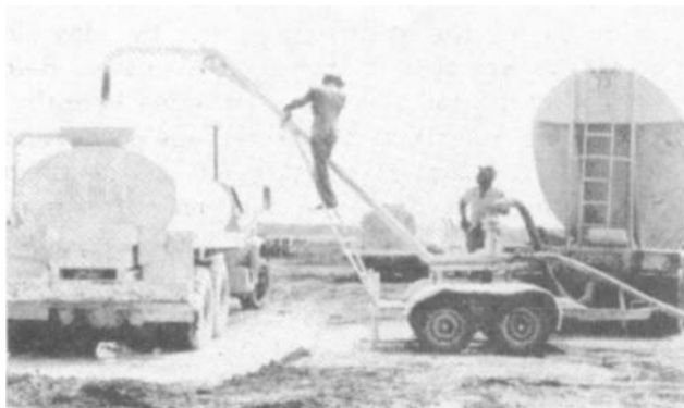
Figure 4-30. Jet slurry mixing plant.
